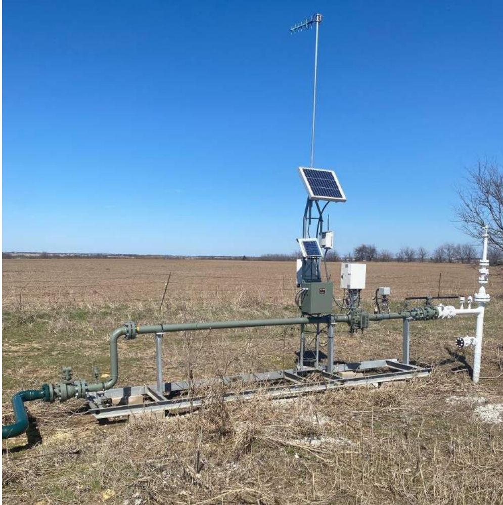
EnLink utilizes solar panels to reduce the need for additional power.
